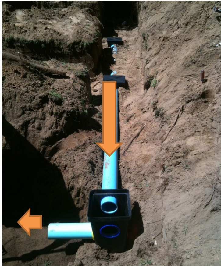
Distributes the effluent from the septic tank to an absorption field located on slopes.
